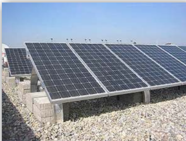
TPM photovoltaic solar power plant
